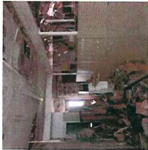
Photograph No. 7 View of rough textured drywall and smooth textured drywall on ceilings.
